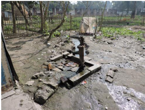
Fig 3.14: Water Supply, Sonatola
