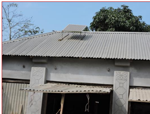
Fig 3.8: Use of Solar Power System
